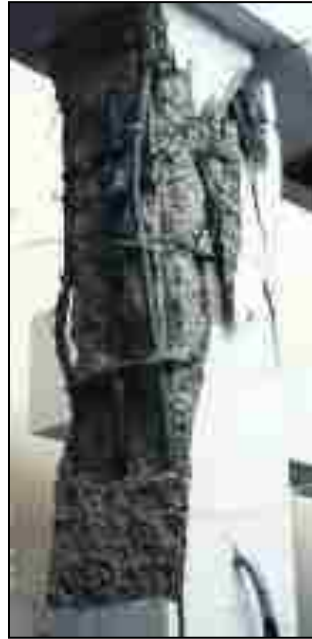
Figure 3.99 Crushing of core concrete: experimental damage (Sezen 2002)
