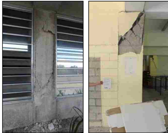
Figures 3.71 and 3.72 Widening and localization of shear cracks: earthquake damage (Eberhard, et al. 2010)
