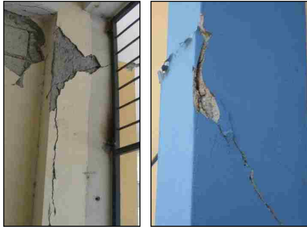
Figures 3.69 and 3.70 Widening and localization of shear cracks: earthquake damage (Sedra, et al. 2010)
