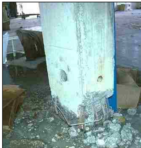
Figure 3.50 Longitudinal bar buckling: earthquake damage (PEER)
