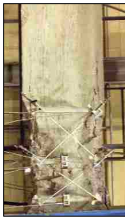
Figure 3.13 (F5) Concrete Spalling Exposing Longitudinal Steel
