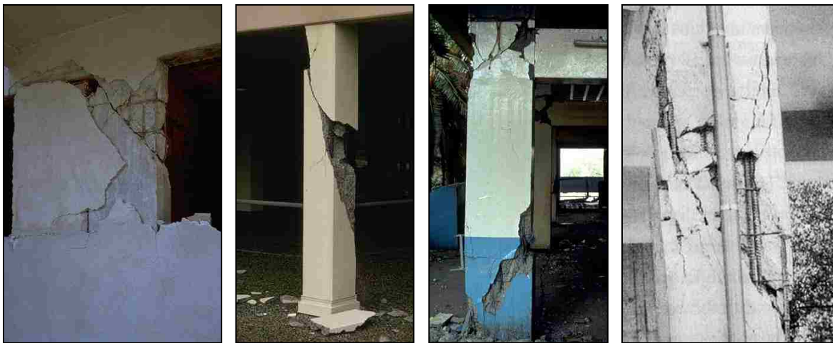
Figures 3.80, 3.81, 3.82, and 3.83 Concrete spalling on side faces: earthquake damage (PEER)
