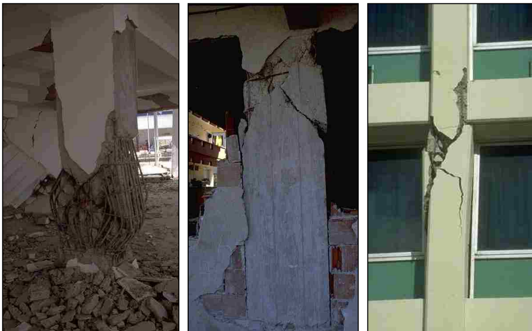
Figures 3.100, 3.101, and 3.102 Crushing of core concrete: earthquake damage (PEER)
