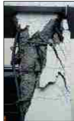
Figure 3.33 (S3.3 & S3.4) Longitudinal Bar Buckling and Core Crushing After Loss of Load Carrying Capacity
