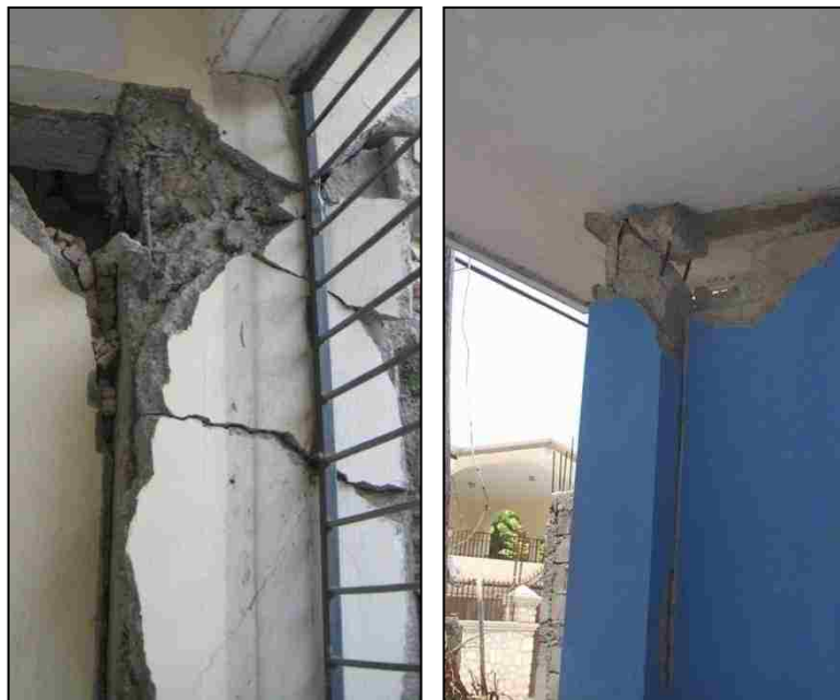
Figures 3.97 and 3.98 Longitudinal bar buckling: earthquake damage (Sedra, et al. 2010)
