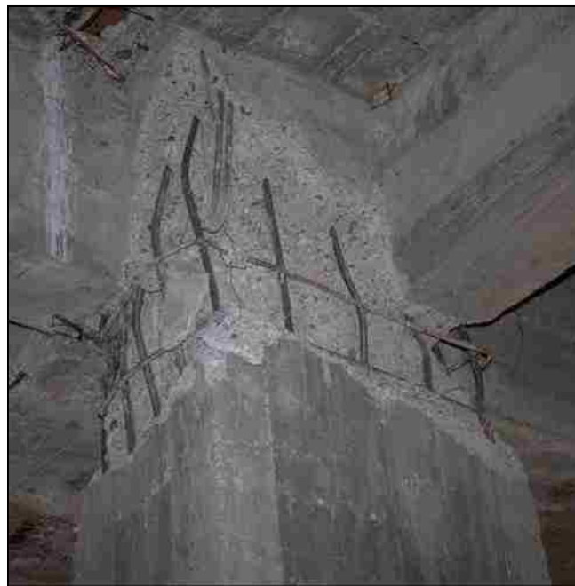
Figure 3.54 Crushing of core concrete: earthquake damage (PEER)
