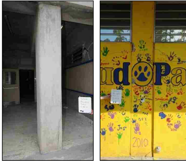
Figures 3.58 and 3.59 Flexural and longitudinal cracking: earthquake damage (Eberhard, et al. 2010)
