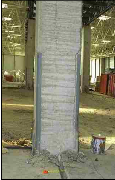
Figure 3.35 Longitudinal cracking: earthquake damage (PEER)
